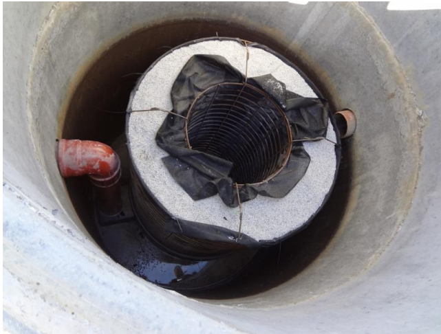
Figure V.8. A cassette with shell sand installed in a drainage well in Denmark to investigate the phosphate sorption capacity of the material. Photo: K. Tonderski, POMInno Sp.zo.o.
